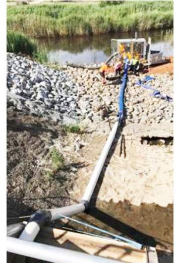
Photo: A temporary pump at East Mirrool Regulator was used in December 2017
