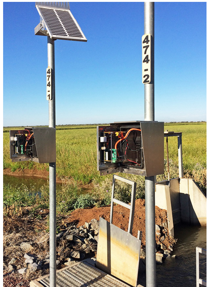
Photo: Recent examples of vandalism and theft to MI infrastructure.
