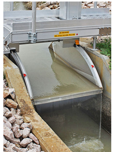
Below: Flume gates at Bilbul are now operating in total channel control mode
