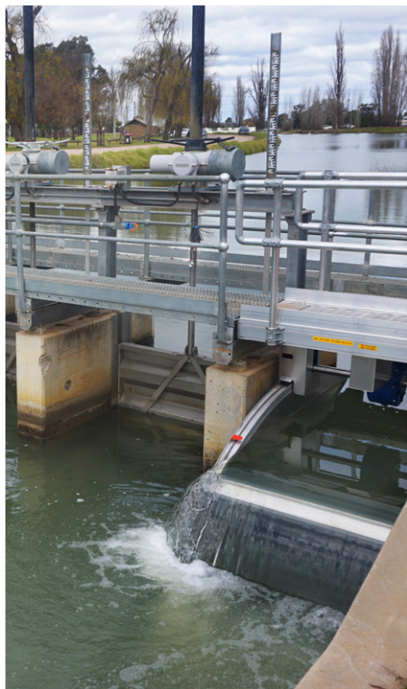
Photo: Upgraded Beltrame's Regulator
