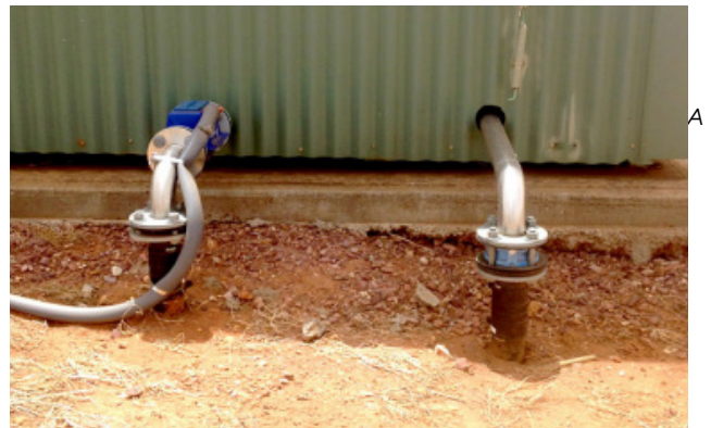
Typical pumping system on farm.
